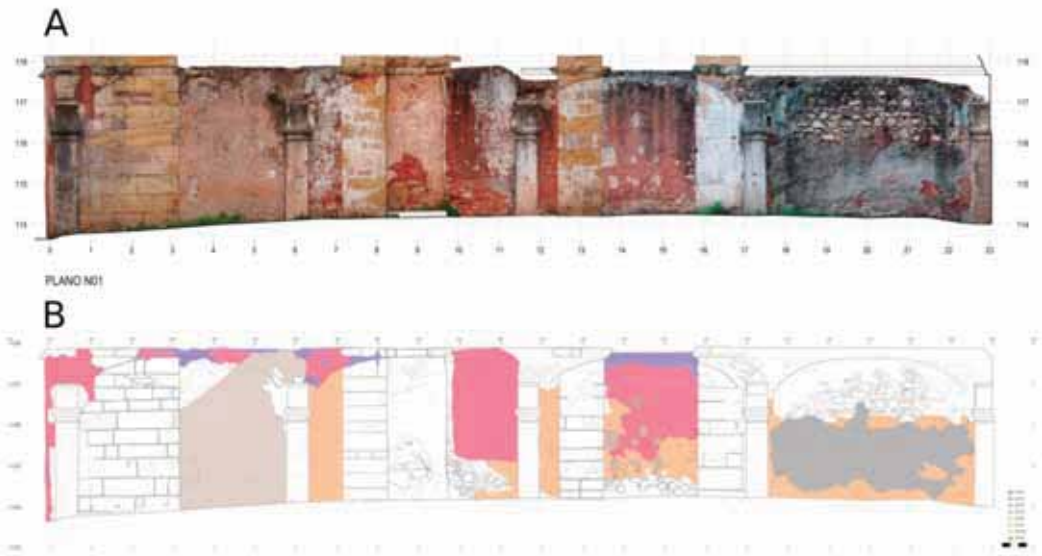
Figure 4. Photo mosaics of the south wall of “Necessárias” (A) and its stratigraphical analysis (B).
